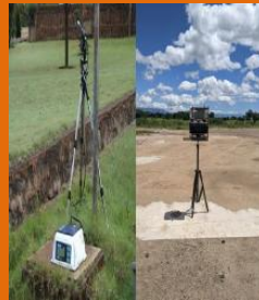
Air Quality equipment monitoring and data collection
